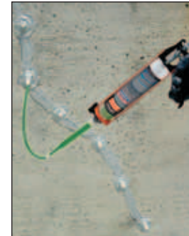
For Leaking Cracks
